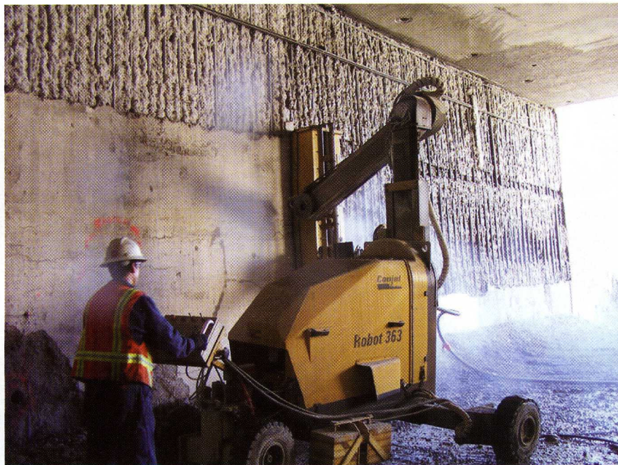
Figure 1: The goal for specialist hydrodemolition contractor on the tunnel walls, which vary in height from about 4.88m to 7.3m, was to cut out damaged concrete to expose to the face side of the reinforcement, but in some areas concrete was selectively removed from behind the reinforcement as a means of inspection.
